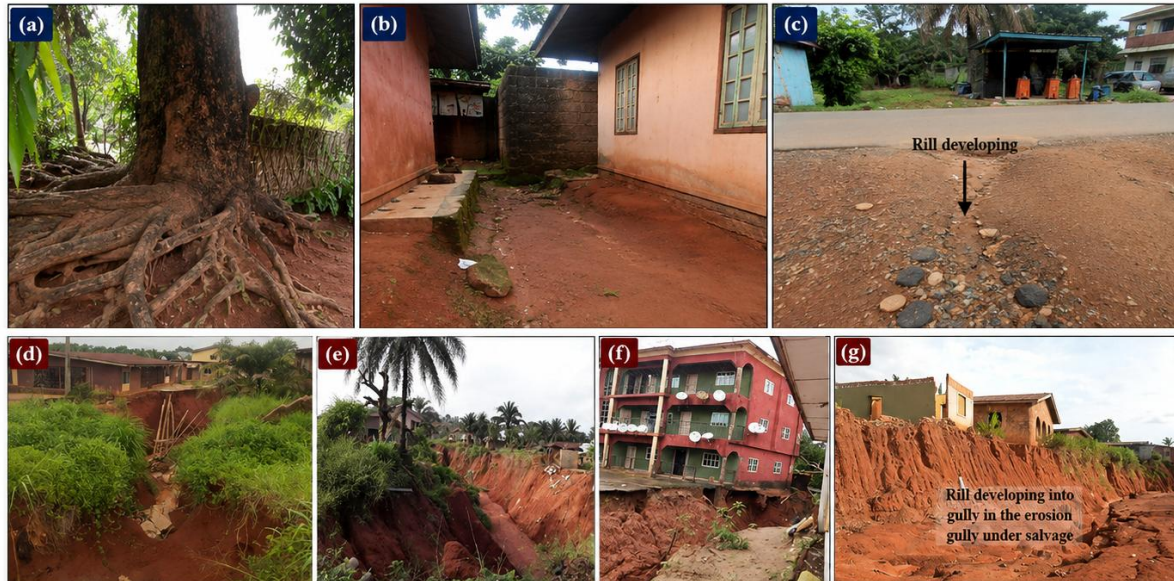
Figure 2. Sheet erosion showing (a) exposed tree roots (b) Exposed house foundation. (c) Sheet erosion developing into rill erosion on an earth road off Odeh Street; (d) and (e) Houses damaged and abandoned due to Midoma/Iweriebor erosion wadi. (f) Damaged and deserted house along Midoma/Iweriebor erosion wadi (g) Damaged and deserted houses on the cliff of Midoma erosion wadi and rill developing into new gully in the erosion gully under salvage.
